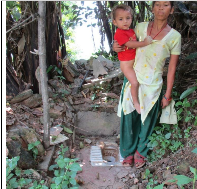
Full damaged toilet
