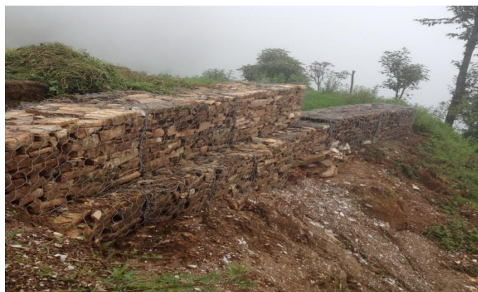
Landslide mitigation in Ghumthang
