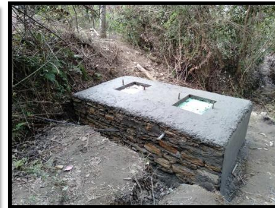
Intake at Luppasing Wafal Bazaar Water Scheme
